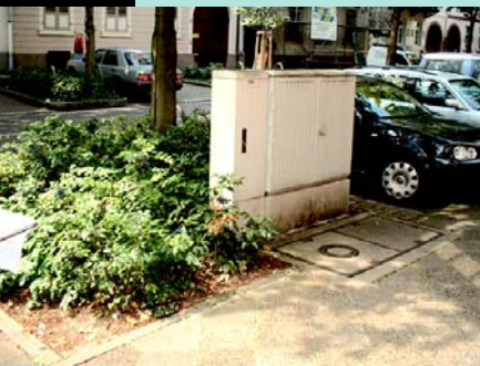
Figure 3 Old distribution cabinet
