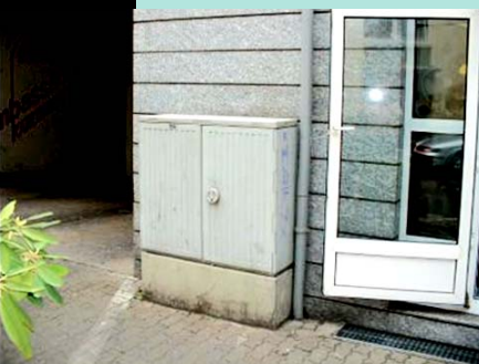
Figure 7 Inconspicuous copper distribution cabinet
