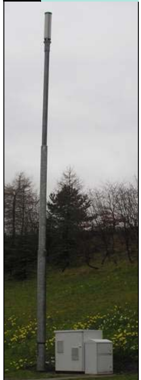
Figure 8 Monopole with collection of cabinets prominent at the roadside
